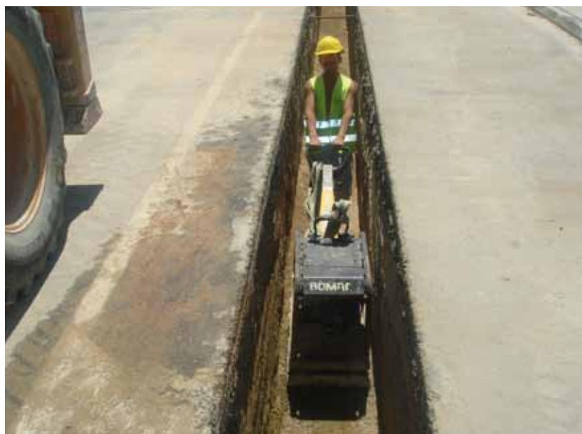
Sewerage system of Kokkinochoria complex (Cyprus)
